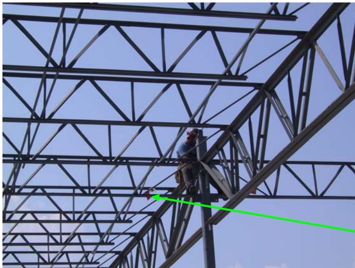
FIGURE 3 COLUMN JOIST BEING CONNECTED; BOTTOM CHORD IS “KNIFED IN” BETWEEN VERTICAL STABILIZER PLATE
