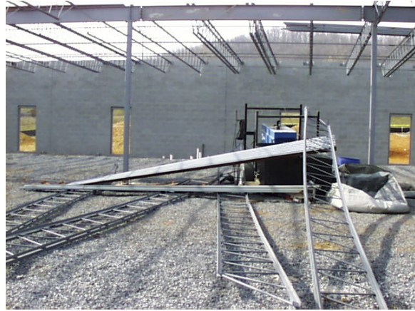
FIGURE 2 POTENTIAL CONSEQUENCE OF SETTING A BUNDLE OF DECK ON UNBRIDGED, UNANCHORED JOISTS
